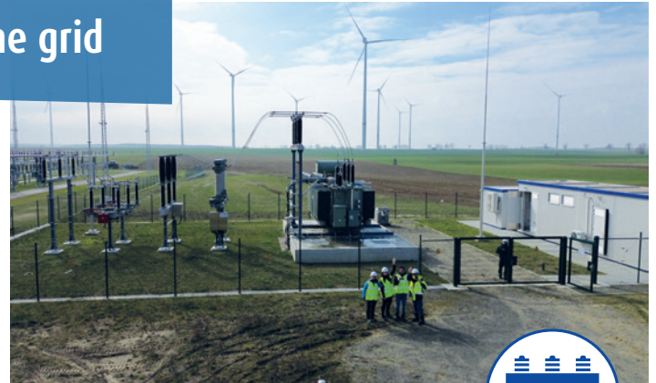
The Wulkow-Trebnitz transformer substation already built
